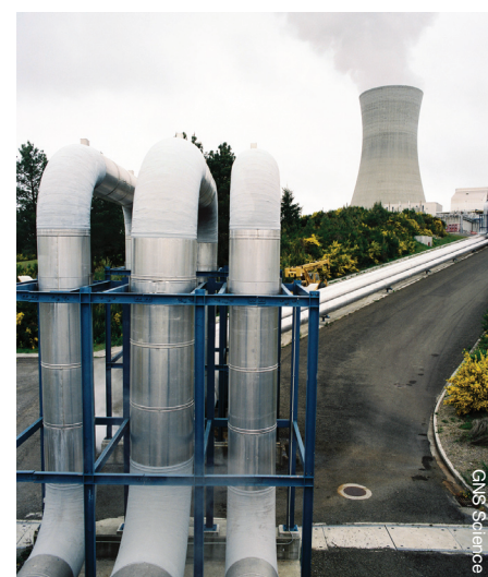
Geothermal power plant
